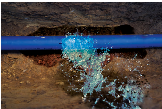
Typical longitudinal crack in a pipe typically caused by earth settlement or increased traffic load.
