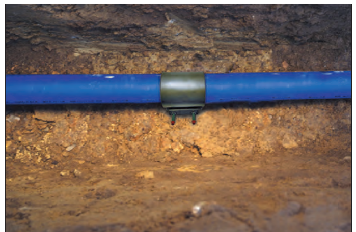
Easy and fast neutralization of the crack is essential in order to minimize disturbance for consumer. Here AVK repair clamp is mounted.
