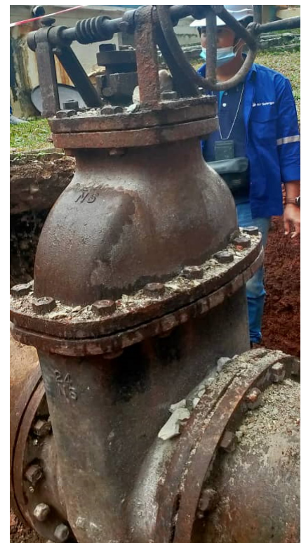
The 95 year-old, fully functional valve, being dug up from the ground in Bukit Nanas, Kuala Lumpur, Malaysia.
