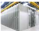
Shanghai Dingyi datacentre
