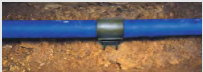
Easy and fast neutralization of the crack is essential in order to minimize disturbance for consumer. Here AVK repair clamp is mounted.
